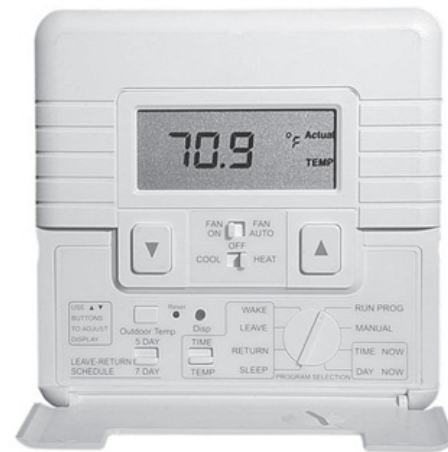
Above: An easy-to-use digital setback thermostat installed by HG&E.
